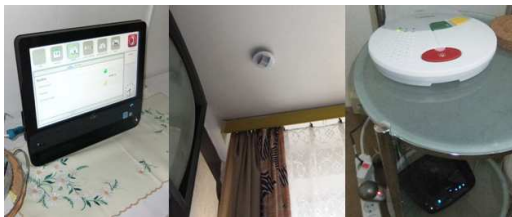
Fig. 1. Residential gateway, presence sensor and social alarm basic unit installed in the user's households (left to right).
